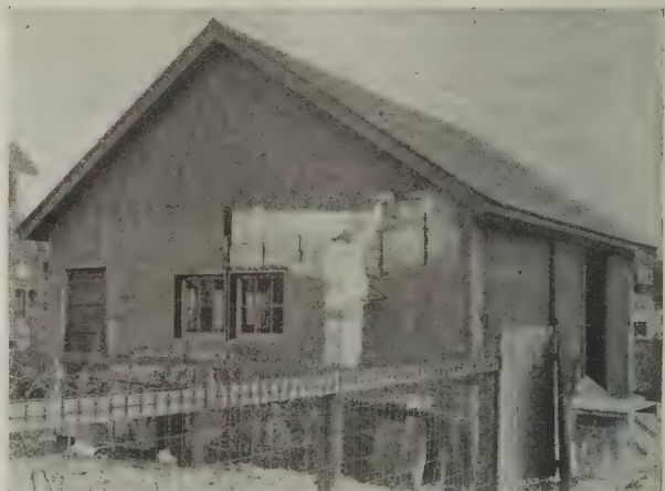
STUCCO GARAGE OF BACK PLASTERED TYPE. IN THIS INSTANCE THE BACK PLASTER WAS APPLIED BEFORE THE EXTERIOR COATS
